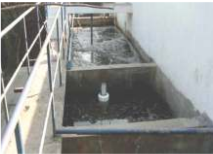
STP Plant for Reuse of Treated water
